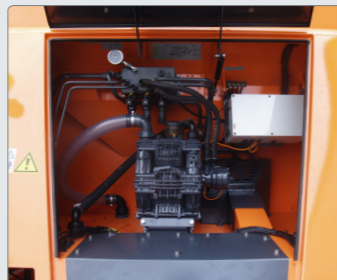
All vital components located together in an enclosed machine room, which offers protection against salt dust. Furthermore, the design has focus on increased user friendliness for drivers and service staff.
